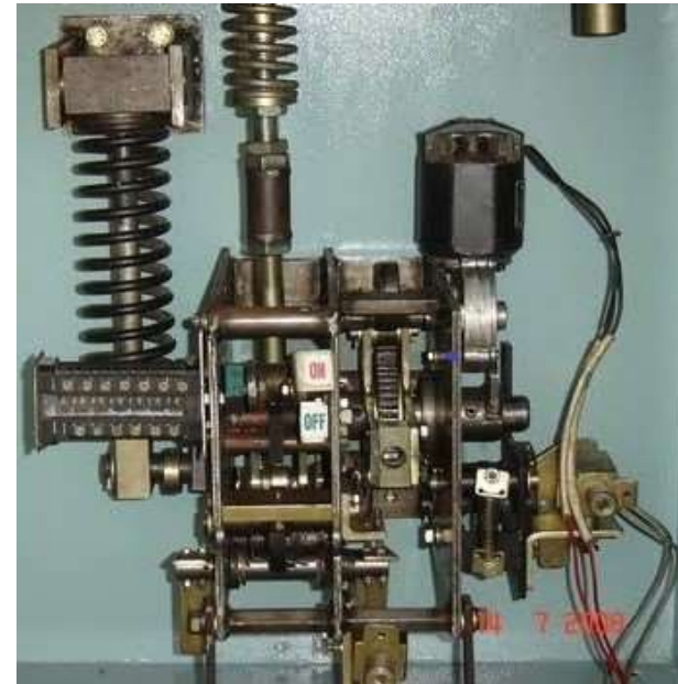
Spring used in circuit breaker
